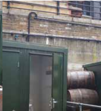
The pipework on the dock wall takes waste from the Saniflo and pumps it up and along the pipes to the main sewer
