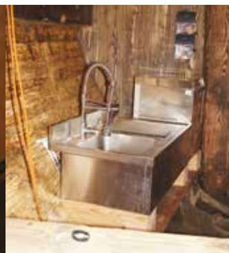
A catering sink with glass washer is plumbed into the Saniflo on board and has a hot and cold water feed
