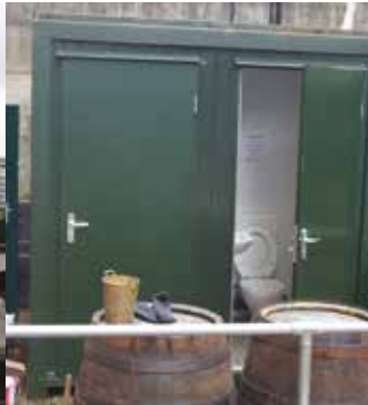
This toilet block in the dry dock connects to the Saniflo that is located directly behind them
