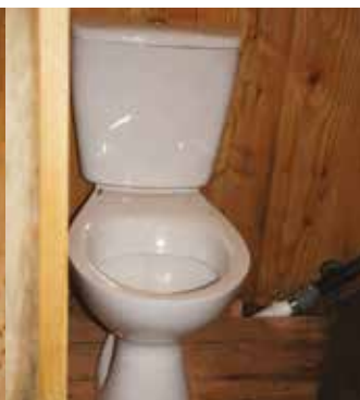
The WC's on board previously had a Saniflo macerator behind each. They now plumb into the Saniflo.
