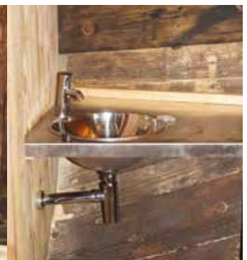
The hand wash basins have been sited separate to the WC to speed up nighttime ablutions
