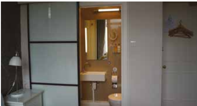
An en-suite was built into a guest room. With no access to mains drains a Saniflo Saniplus macerator takes the waste away.
