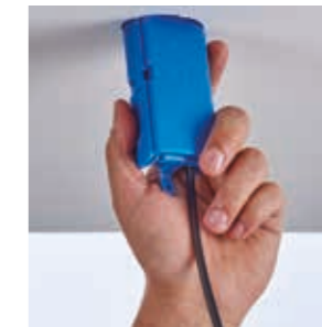
Simple spotlight installation
