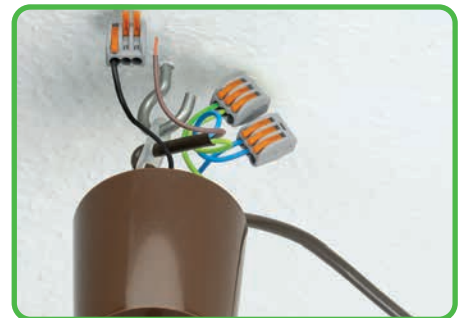
Lighting fixture connected with flexible power feed.
